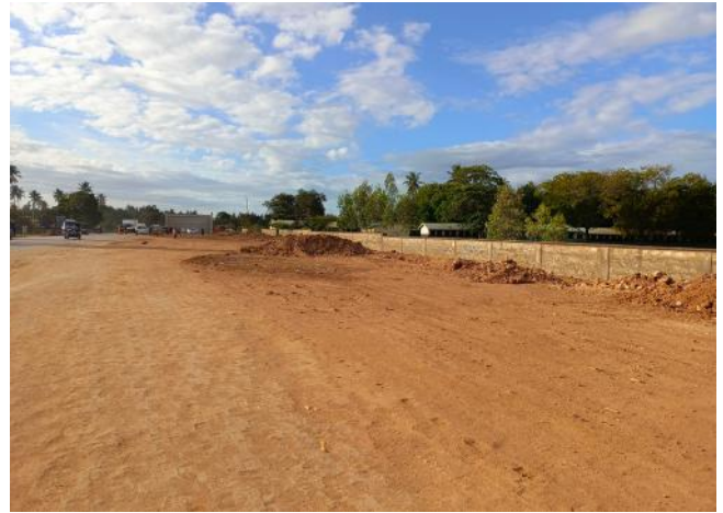
Road construction soil heap moved by KeNHA after Shimo La Tewa Primary School learners complained of lack of a designated and clear footpath to walk on.
